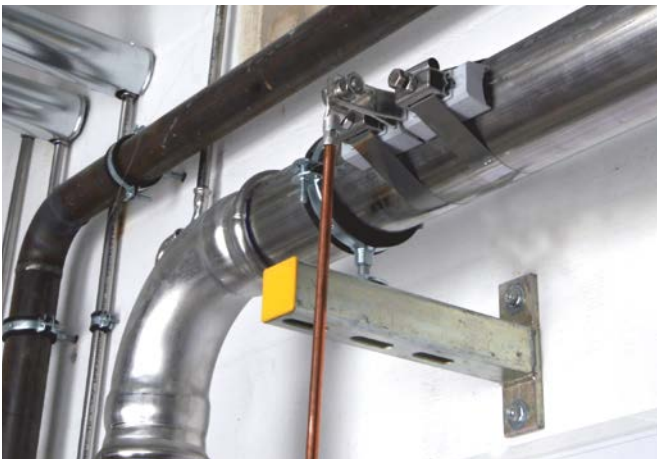
Installed at a StSt pipe.
