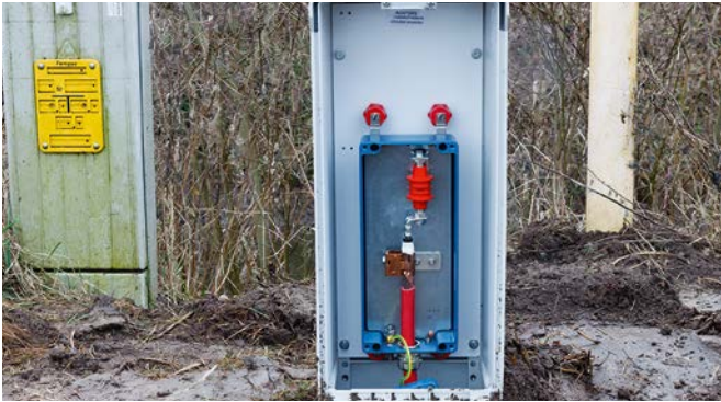
Coaxial connection of the Ex isolating spark gap for protecting buried insulating joints
