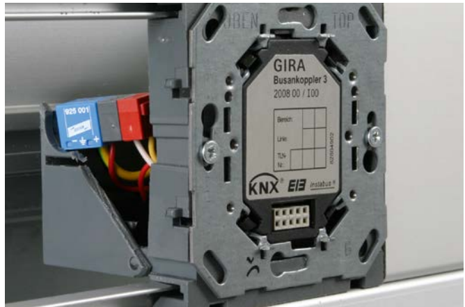
Protection of a KNX bus coupling unit by means of a BUSector surge arrester mounted on a bus terminal in the mounting panel of a cable duct.
