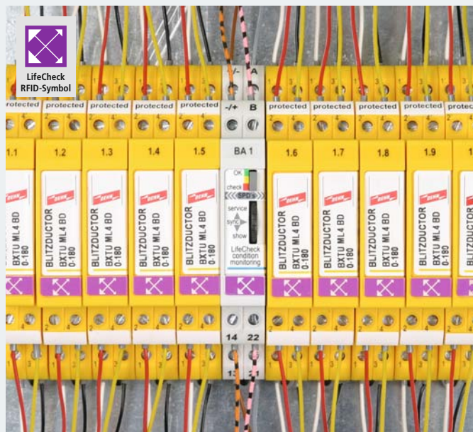
DEHRecord Condition Monitoring Einheit in der Installation.
